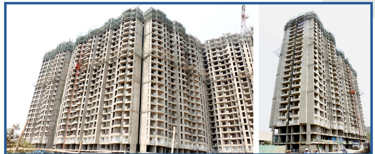
JP NORTH Estella | MAHARERA No: P51700008916 • Building structure completed • Overhead water tank structure completed • Underground water tank in progress
