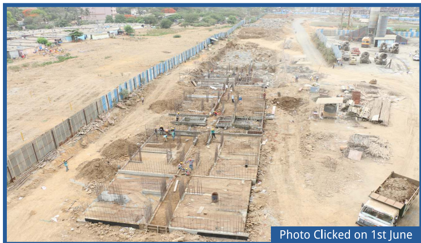
JP NORTH Elara | MAHARERA No: P51700007001 • A wing footing and column completed • B wing footing in progress • C Wing excavation completed
