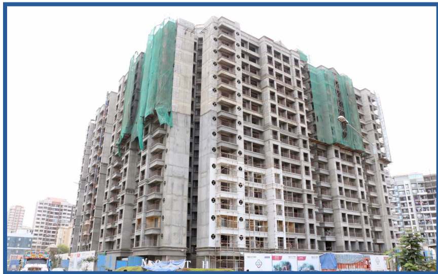
JP NORTH Celeste | MAHARERA No: P51700008667 • Building structure completed • Underground water tank in progress • Overhead water tank structure completed
