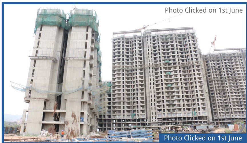
JP NORTH Atria | MAHARERA No: P51700004117 • 3A-11 slabs completed, 12 work in progress • 3B-12 slabs completed, 13 work in progress
